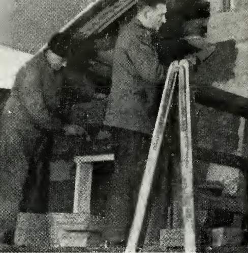
Brother Stone and President Aubrey lay bricks to aid the Hull Branch building project.
